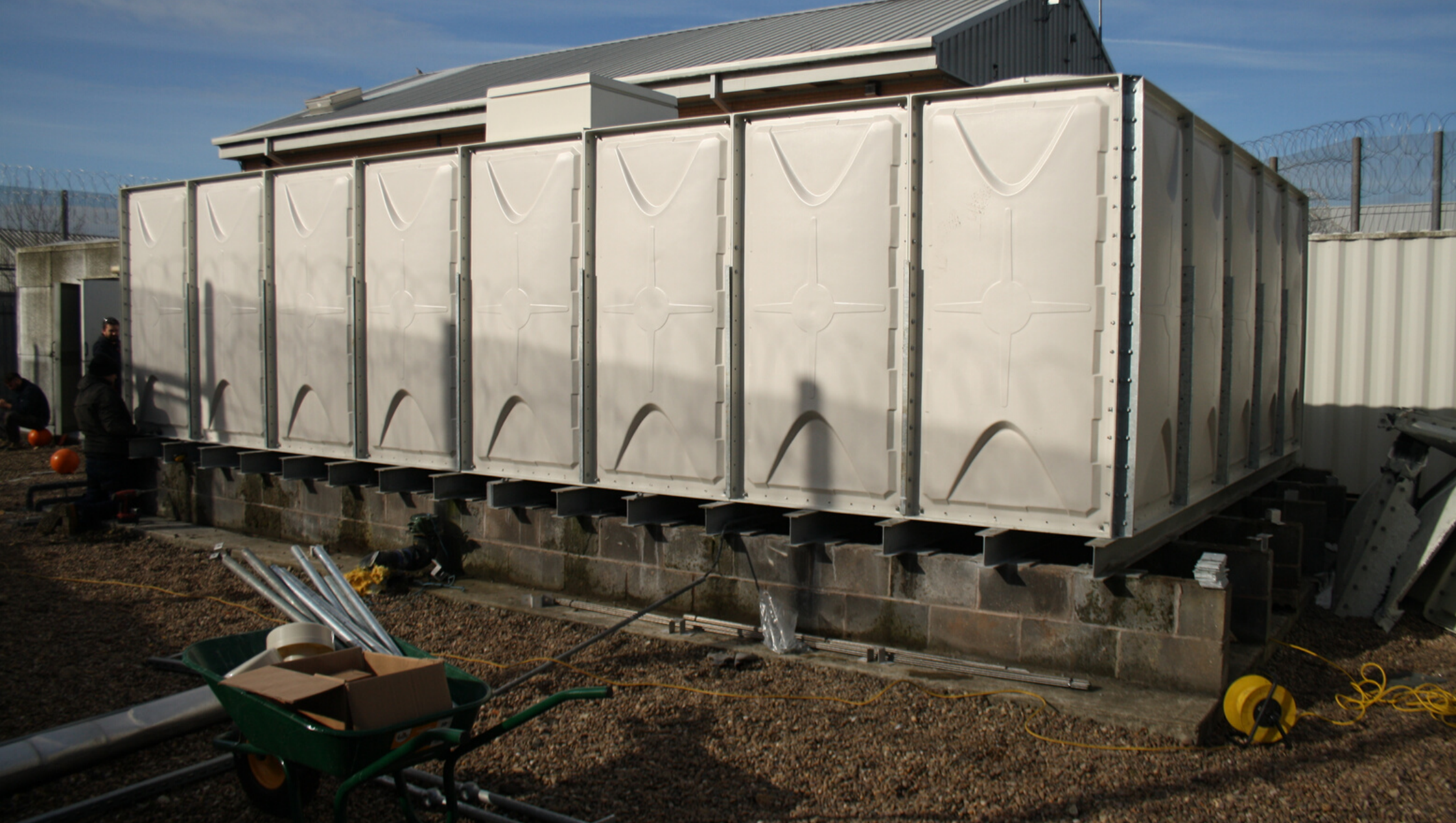
AN EXAMPLE OF A 8X5X2 METRE GRP WATER TANK REPLACEMENT CARRIED OUT AT A SECURE FACILITY IN THE UK
