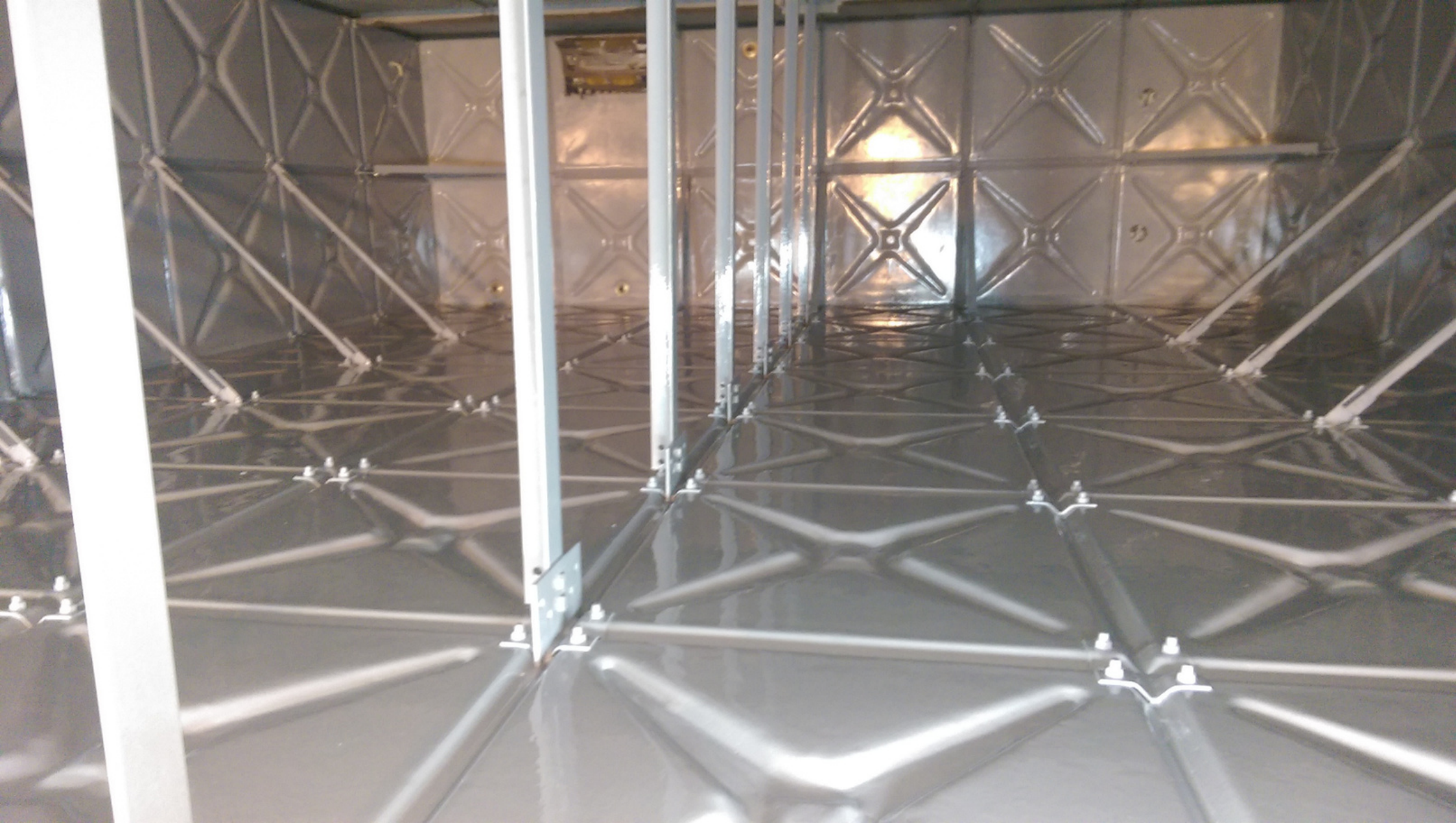
AN EXAMPLE OF OUR SPRAY APPLIED POLYUREA, INSTALLED IN A LARGE STEEL BRAITHWAITE TANK IN A HOSPITAL IN YORKSHIRE
